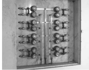
Original 1914 fuse box with asbestos liner
